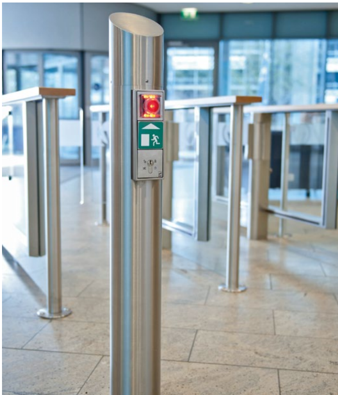
Card reader post with escape route terminal
